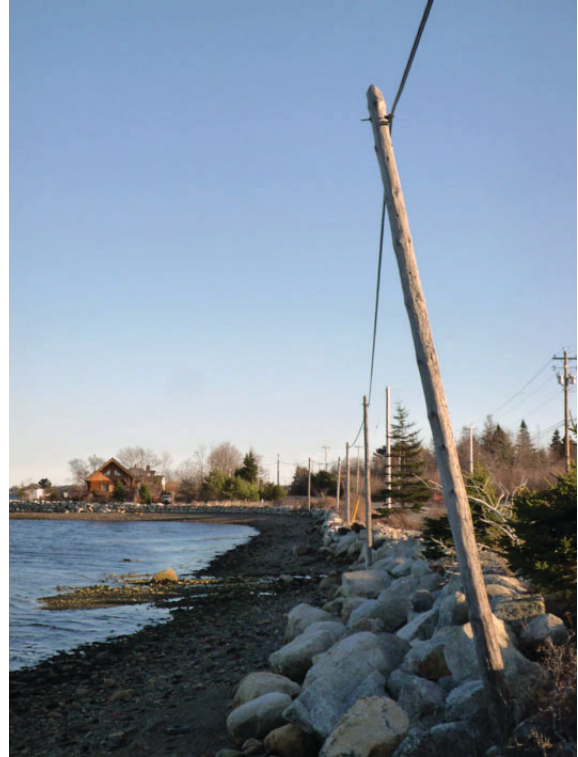
Figure 13: vulnerable utility poles in Western Shore.
