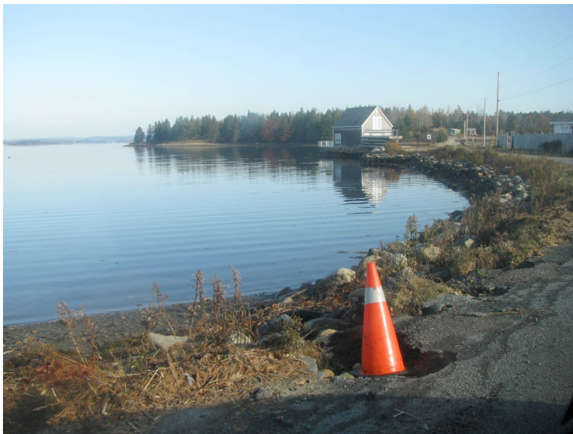
Figure 4. A photograph of the road damage leading to the Oak Island Causeway, which was caused by increased storm surge that was brought in by a nor'easter. Photo: Mirjam Held.
