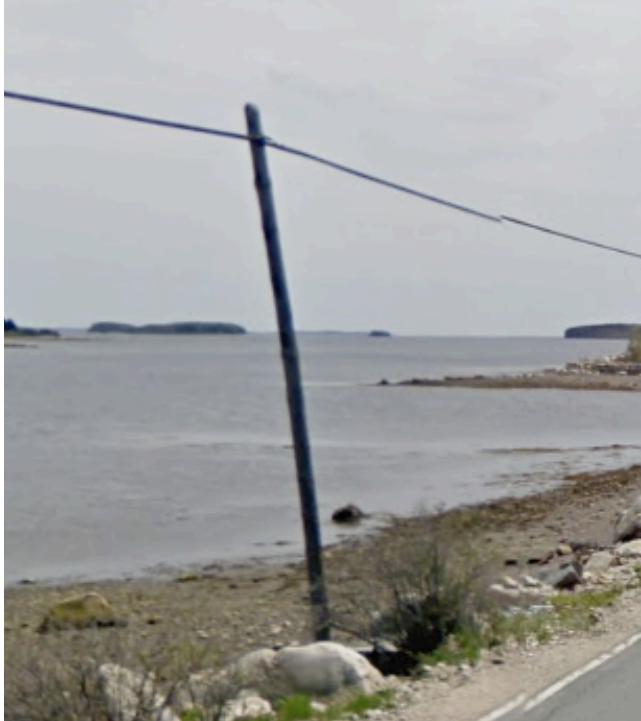
Figure 8. An example of one of the power poles that has its base covered by water at high tide.
